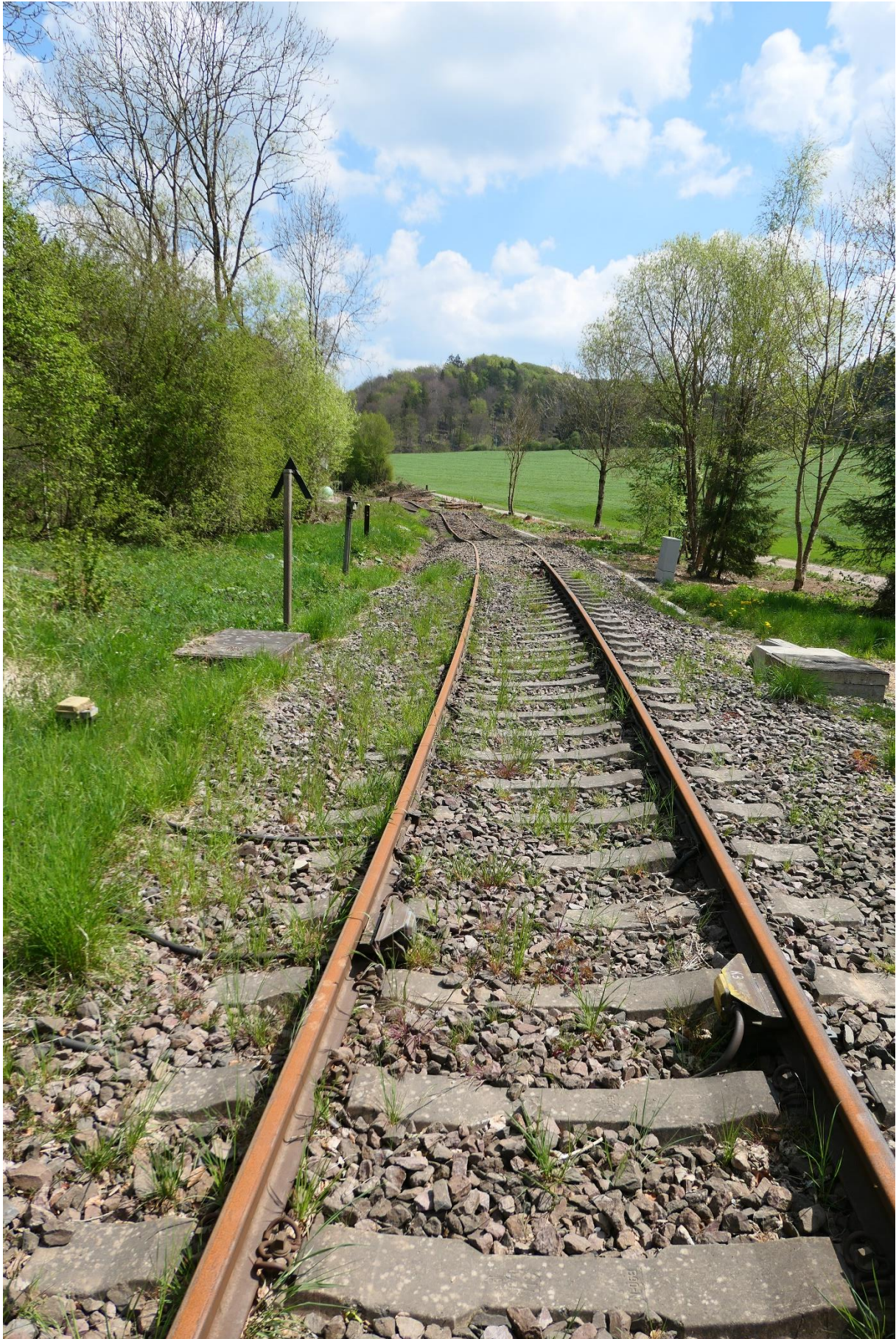
The Urft valley railway looking worst for ware after the 2021 floods.
